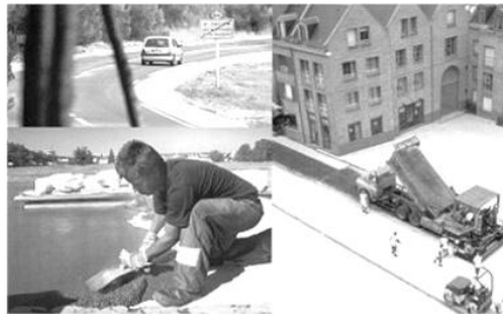
Fig. 2. – The methodology most often applied is the preparation and manual cast of coloured asphaltic mixtures, especially in small-sized places.
