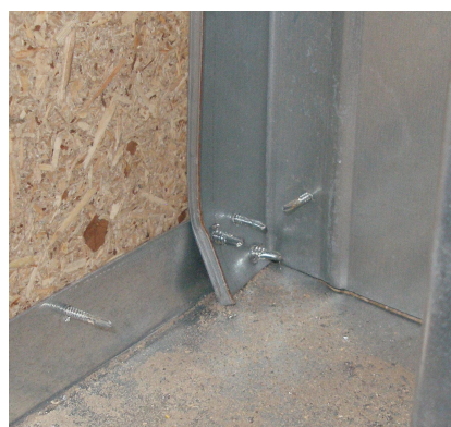
Fig. 14. – Deformation of the vertical steel profile at the corner of the structure.
