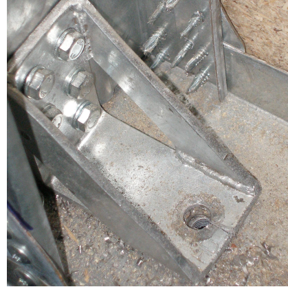
Fig. 16. – Breaking of the anchorage bolt and of the corner steel piece.
