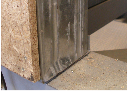
Fig. 15. – Local deformation of the lower left steel profile of the door frame.
