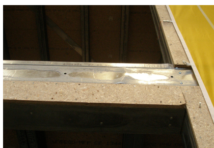
Fig. 13. – Local buckling of the frame girder at the level of the first floor.
