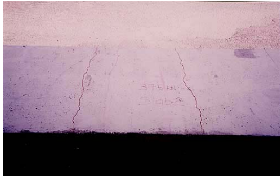
Fig.4 a – Crack pattern before repair.
