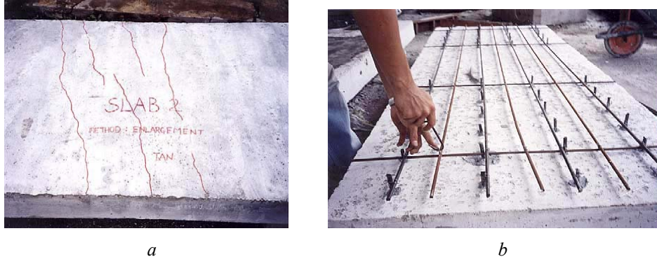
Fig.6 – Strengthening by enlarging the slab section: a – crack pattern before repair; b – roughened surface and steel provided.
