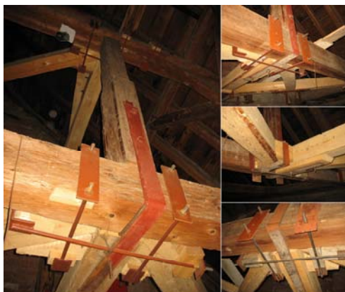
Fig. 1 – Case studies for strengthening works of beams and columns using traditional materials and methods.
