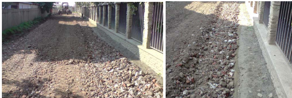
Fig. 7 – The effect of 150...300 mm broken cement concrete on the uniformity of the constructed layer.
