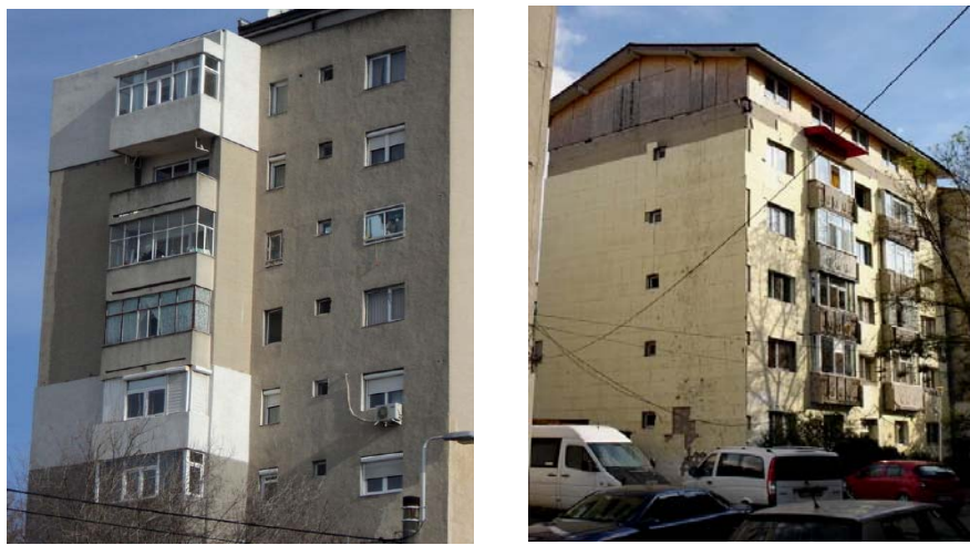
Fig. 2 – Execution of a partial insulation with EPS of buildings or improper execution (Constanța – Romania).
