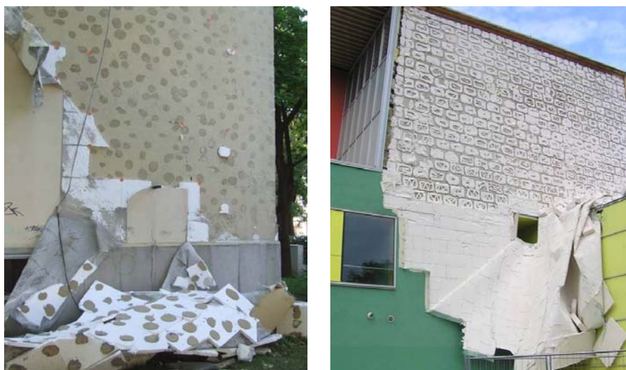
Fig. 3 – Partial or total detachments of the thermal insulating system from the resistance structure.
