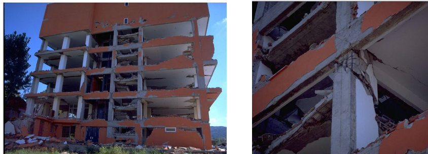
Fig. 1 – Damaged RC frame with hollow clay tile infill masonry, Izmit 1999 (Elwood et al. , 2000).
