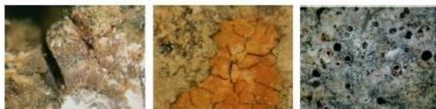
Fig. 3 – Physical (first image on the left – cracks of the material) and biological (images from the middle and on the right) degradations, investigated with the FOM technique (Moropoulou et al. , 2013).
