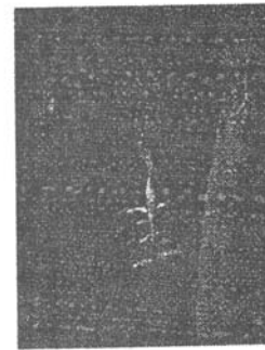
Fig. 9.- The steel joint failure - vertical crack in joint panel near horizontal stiffener.
