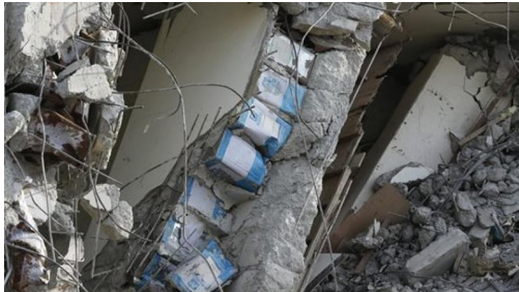
Fig. 6 – Cans in the structural walls of the collapse building in Taiwan, 2016.
