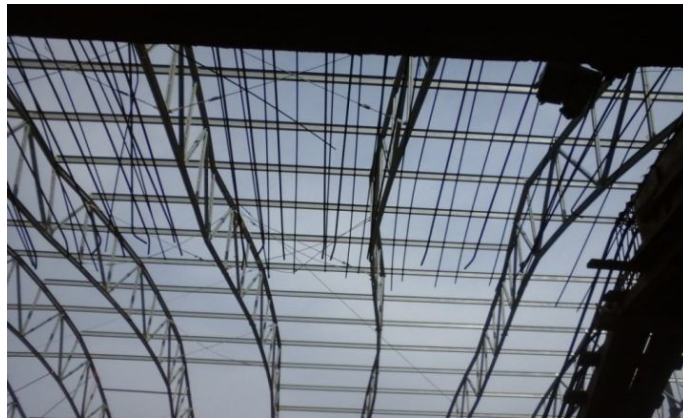
Fig. 2 – Truss arches roof system assembly without assuring lateral stability of the elements.
