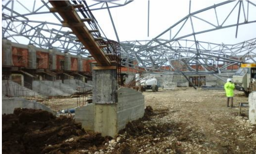
Fig. 3 – General collapse of the roof system.
