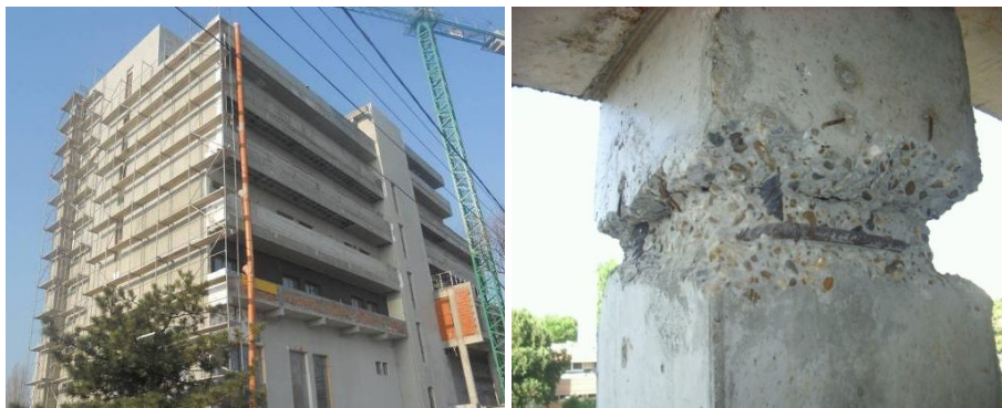
Fig. 7 – Damage structure due to sawdust in the ground floor columns.
