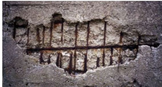
Fig. 15 – Spalling of concrete due to sulphate attack.
