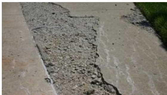
Fig. 11 – Concrete affected by freeze-thaw cycles.
