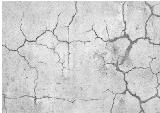
Fig. 5 – Drying shrinkage due to poor curing.
