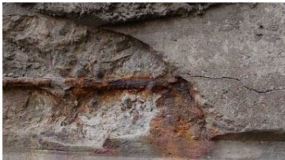
Fig. 10 – Concrete affected by alternate wetting and drying.
