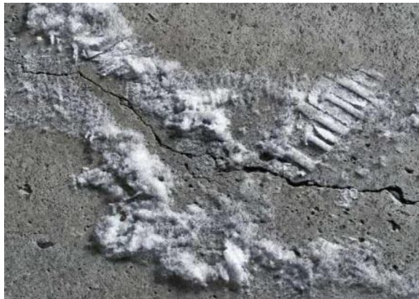
Fig. 8 – Efflorescence in concrete.
