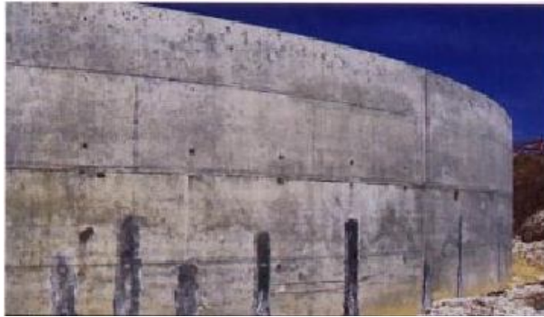
Fig. 6 – Thermal cracks in concrete.
