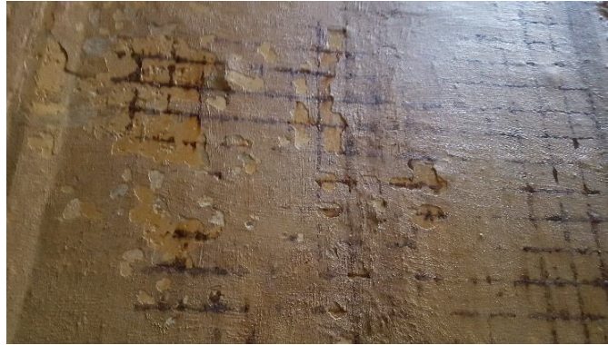
Fig. 14 – Corroded reinforcements at the level of the water tank wall – Miroslava commune, Iași County.
