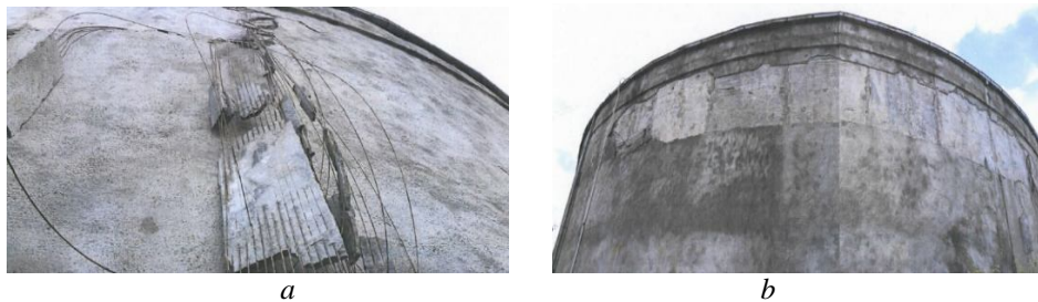
Fig. 4 – Degradations at the top of the water tank wall.
