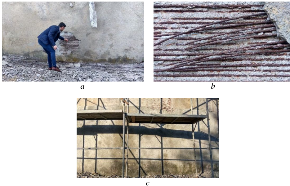
Fig. 5 – Degradation at the base of the water tank wall.
