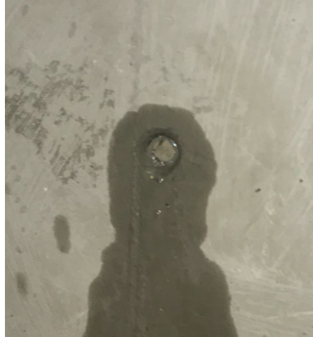
Fig. 5 – Incorrect use of the tubes doppers for sealing realization in the joint zones.
