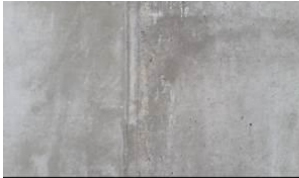
Fig. 2 – Demolded concrete of the reservoir wall – TEGO frame work – left; metallic frame work – wright.
