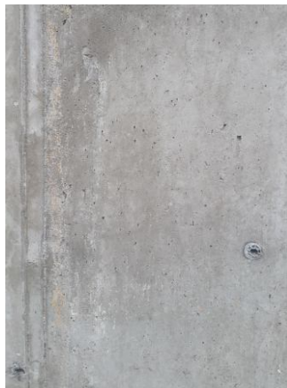
Fig. 3 – Demolded concrete of the reservoir wall – zone of passing for joint elements.
