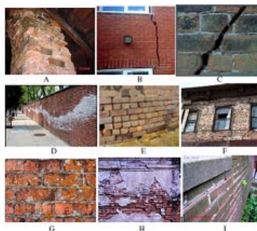
Fig. 1 – Damage encountered in masonry:
