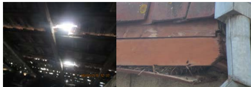
Fig. 3 – Elements of damaged roof framing, Damaged, broken eaves and pipes.
