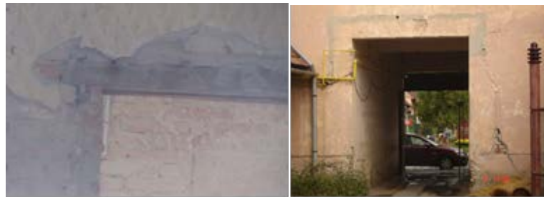
Fig. 11 – Damage at the door void. Ground floor walls with fissures and cracks.
