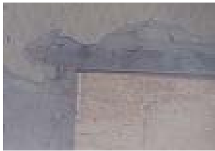
Fig. 6 – Damage at the door void.
