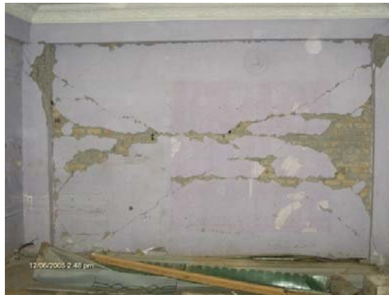
Fig. 1 – Masonry panel cracked due to horizontal seismic action (Javed et al. , 2006).
