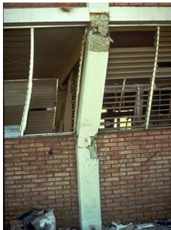
Fig. 3 – Failure mechanism due to short column development (Pradhan et al. , 2012).
