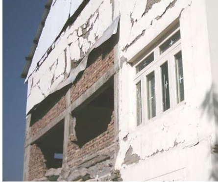
Fig. 2 – Masonry panel expelled from the structural system (Javed et al. , 2006).
